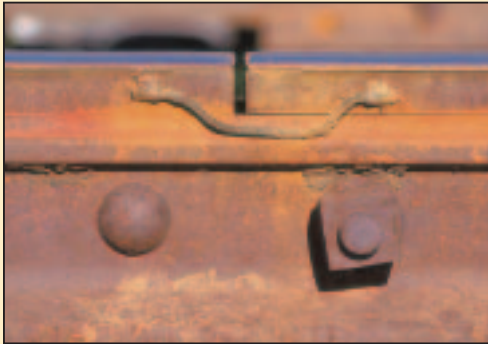
Figure 2.19a) Train tracks span great distances. Spaced many metres apart are small gaps between the rails. What's the purpose of these gaps? What might happen if the gaps weren't there?
